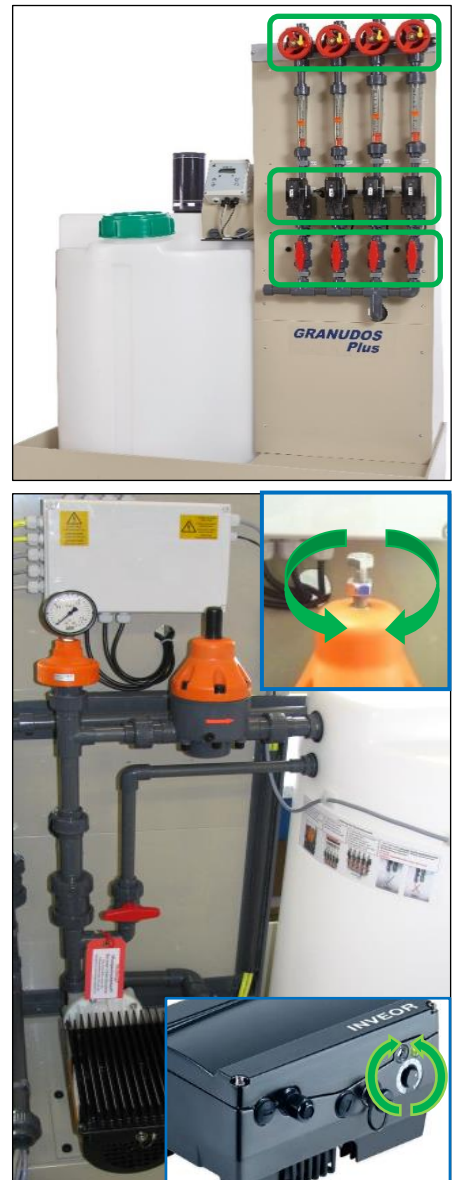
Figure 29, Distribution system, pressure retention valve, frequency converter
